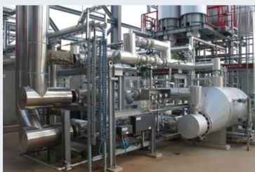
Hot Oil / Water Transfer
